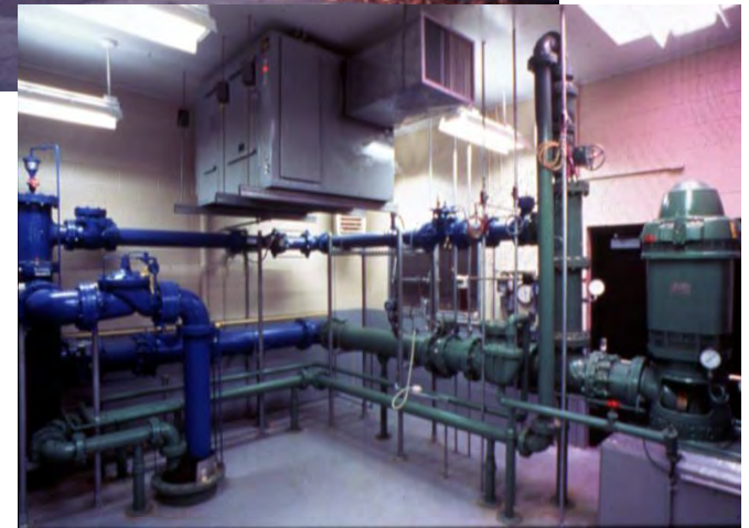
Murray Avenue ASR Well Cherry Hill, New Jersey
