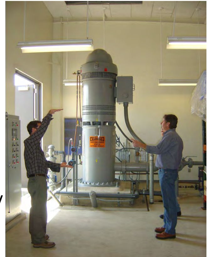
Calleguas MWD, California
