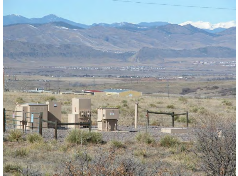
Highlands Ranch, CO One of 26 ASR wells underground in vaults
