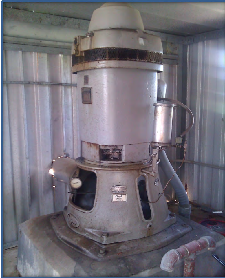
Figure 4: Well Pump at Station 21
