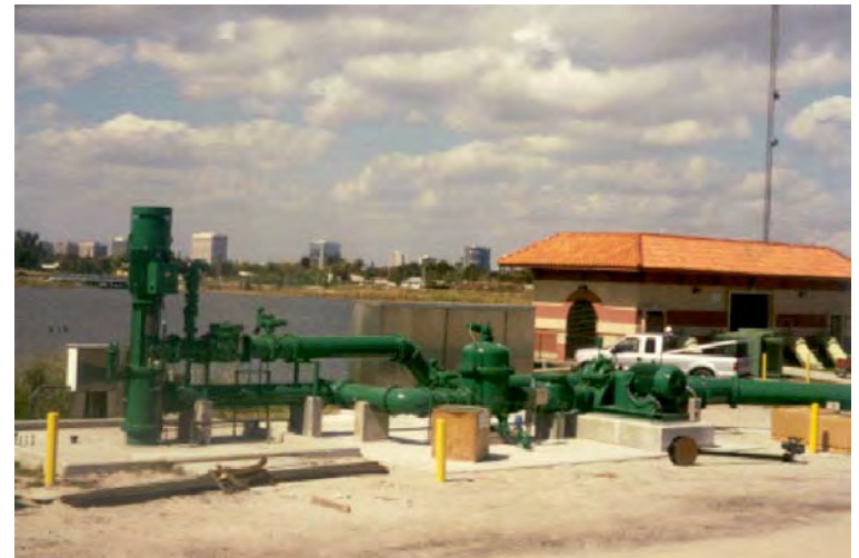
West Palm Beach, Florida ASR Well – 8 MGD Capacity Largest ASR Well in the World
