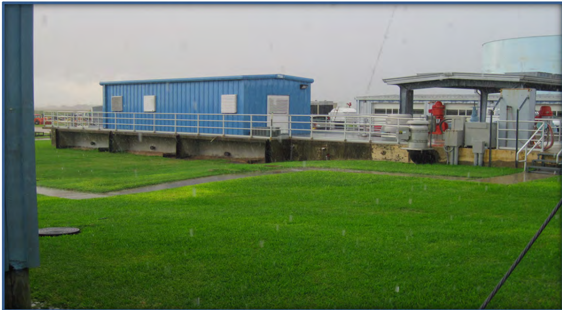
Figure 7: PLWTP Filters and Transfer Pumps
