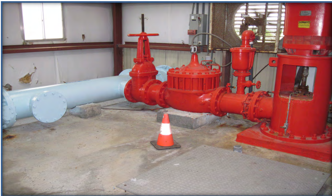
Figure 8: PLWTP HSPS Showing Spare
